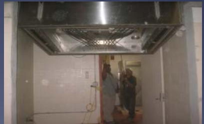
4. View of heater plenum
