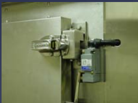
Door latch and cut-off switch
